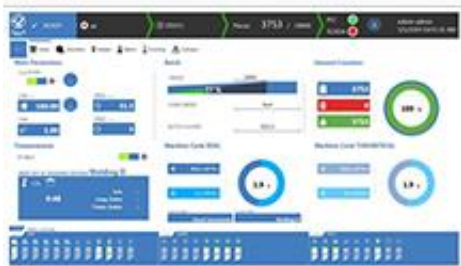
Controls & User-Interface Upgrades
